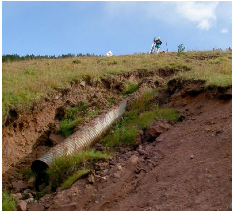
Failing fill slope culvert
