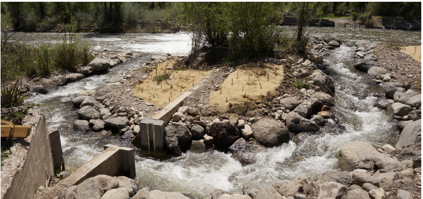
Elk Creek Fish Passage channel around the Ware and Hinds Diversion Dam in New Castle, CO
